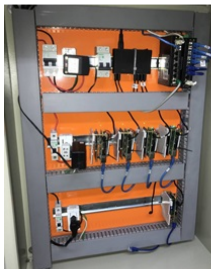
Figure 15. Supervisory system hardware box.
