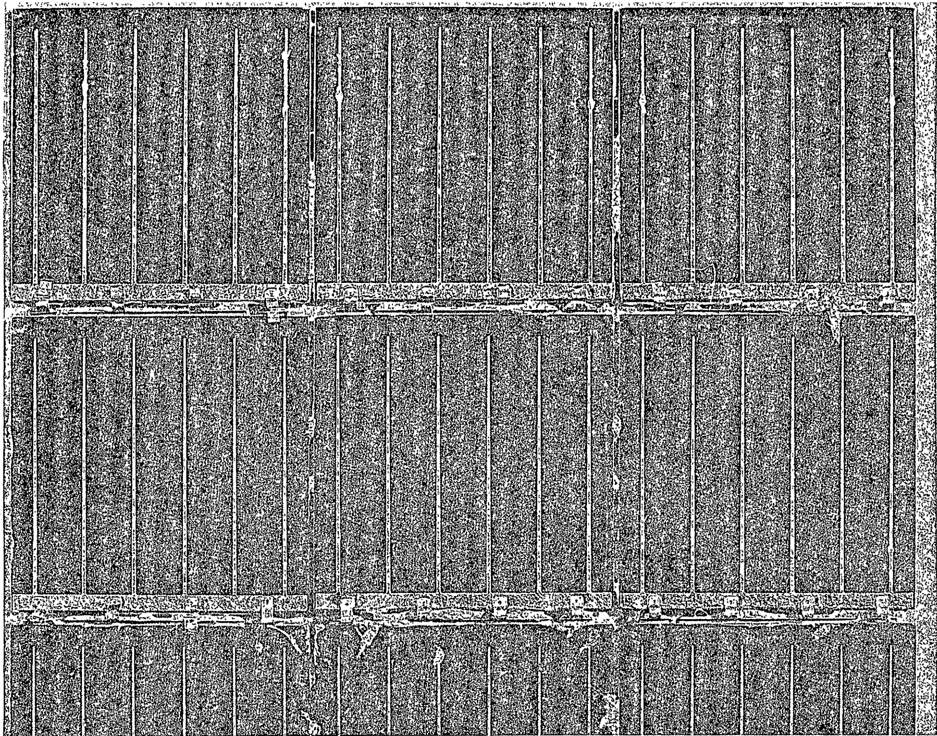
FIGURE 2-3-11. Z TAB FAILURE
