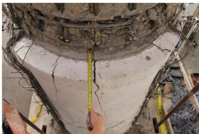
Fig. 10. Cracks atop of the pile of Specimen 4
