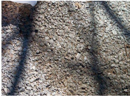
Figure 2.16: Clogged Pervious Concrete Pavement
