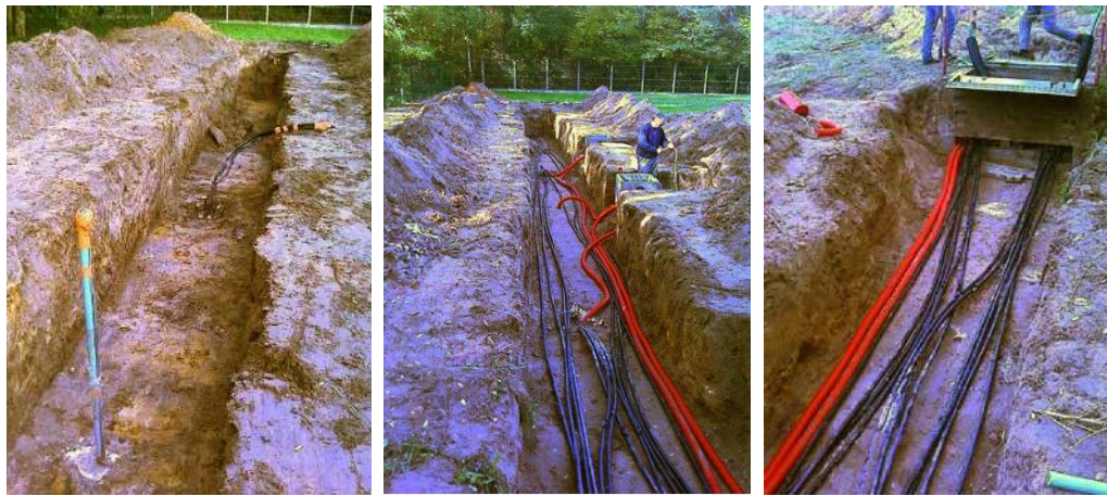
Figure 4.7: Sensor cable cutting and connecting to the manifold well (here, red pipes contain the sensor cables)
