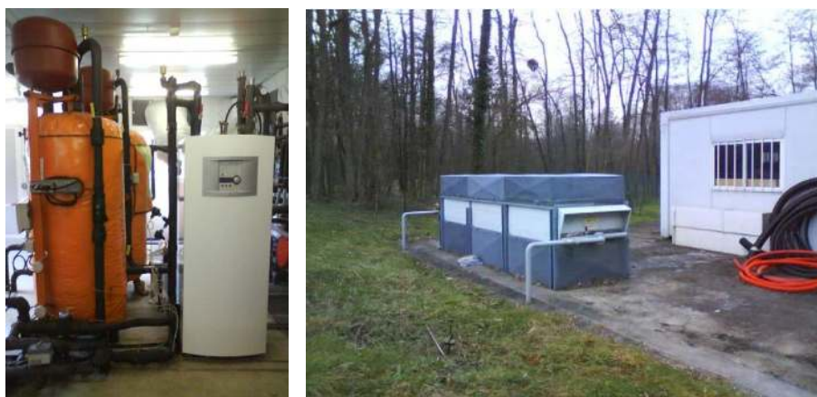
Figure 4.3: Heat pump and second water loop with 500l water tanks (left) and Air cooler (right)
