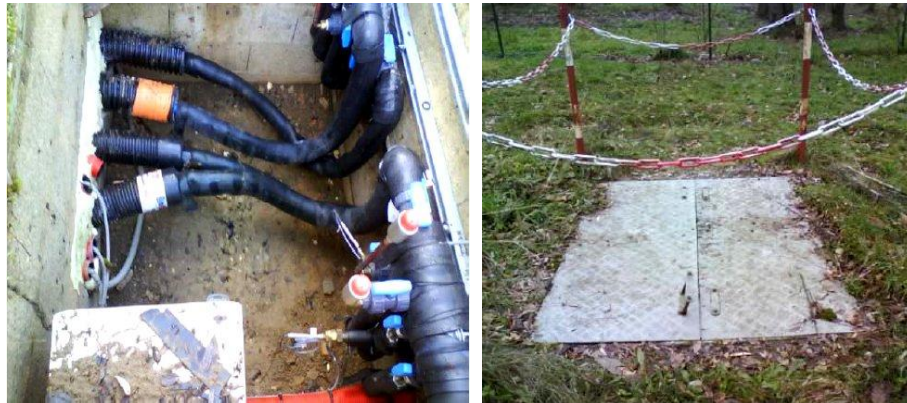
Figure 4.9: Manifolds and Temperature sensors (left) and Metallic cover of the manifold well (right)
