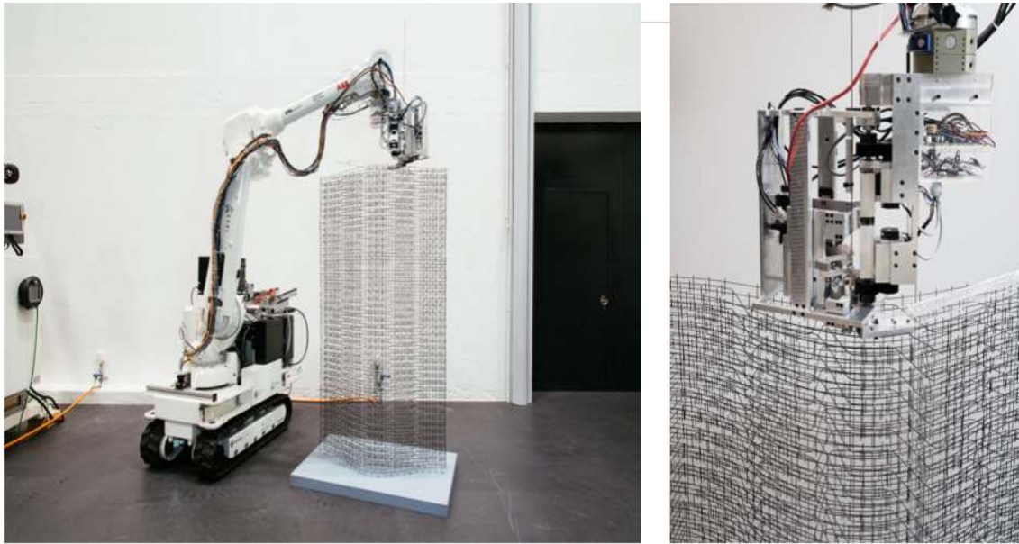
Figure 2. (Left) Mesh Mould produced with the In Situ Fabricator robot from ETH Zurich dfab. (Right) Close up of In Situ Fabricator tool head.
