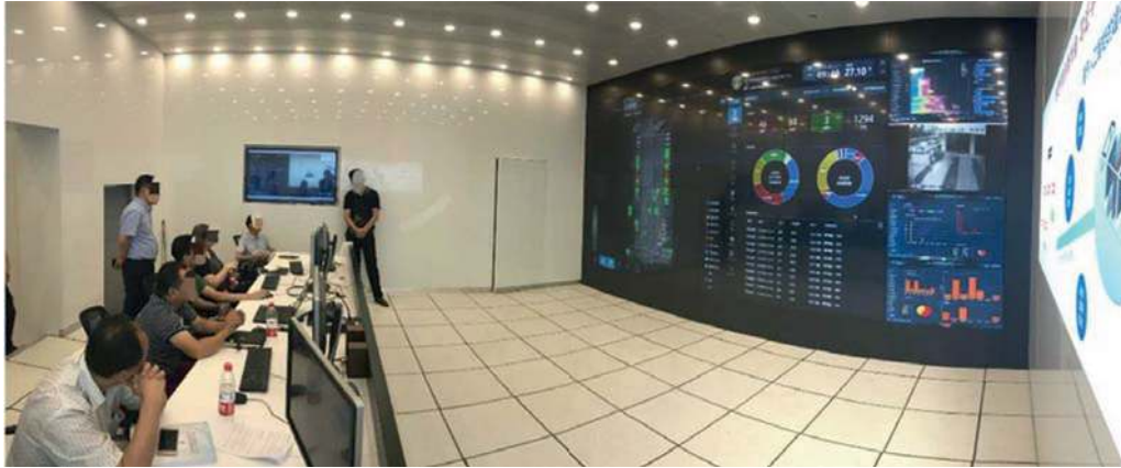
FIGURE 5: The main hall of the DT control center.
