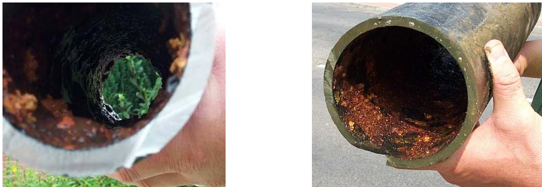
Fig 1-4 Material accumulation around the complete perimeter of cast iron pipe samples
