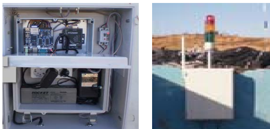
Fig. 3. Interior and exterior of sensor logger system.
