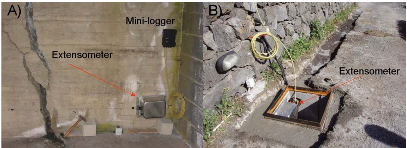
Figure 3. Photographs of the Et1 (A) and Et2 (B) extensometer sites during installation.
