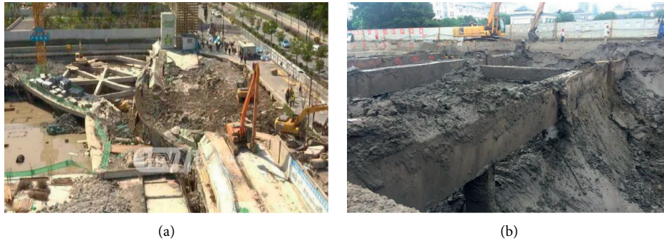
FIGURE 1: Foundation pit accidents: (a) foundation pit collapse and (b) the sudden surge of foundation.
