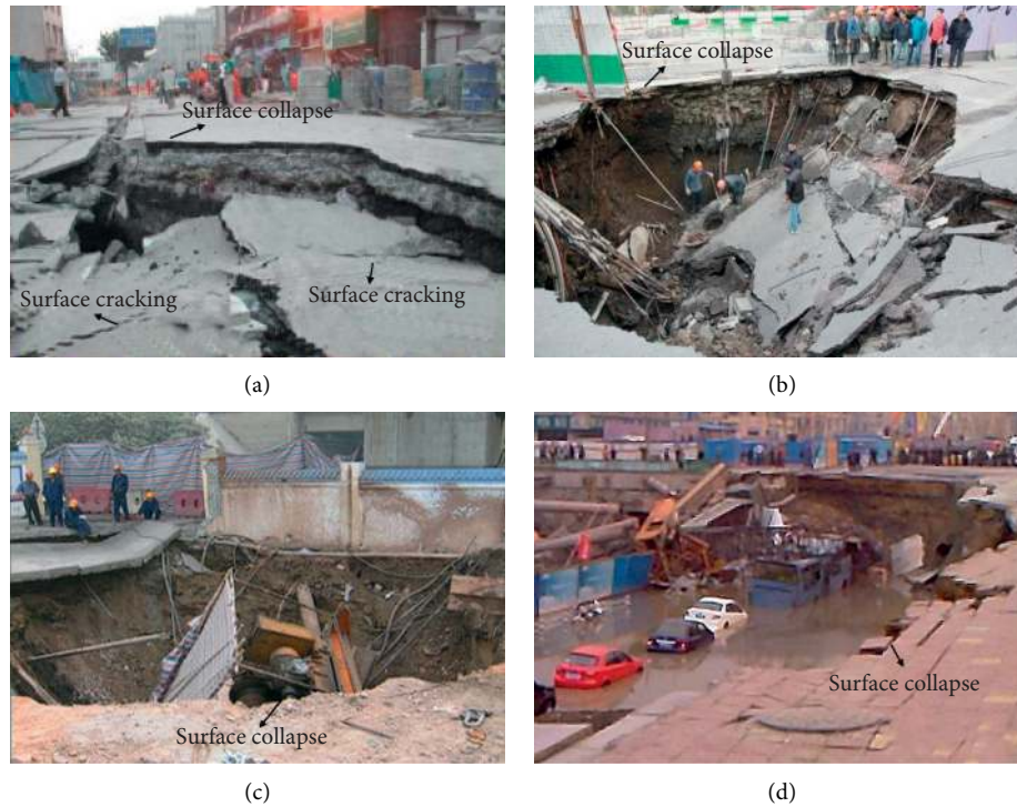
FIGURE 1: On-site photos of surface collapse and surface cracking. (a) Shanghai metro line 4, (b) Nanjing metro, (c) Guangzhou metro line 5, (d) Hangzhou metro line 1 [29].
