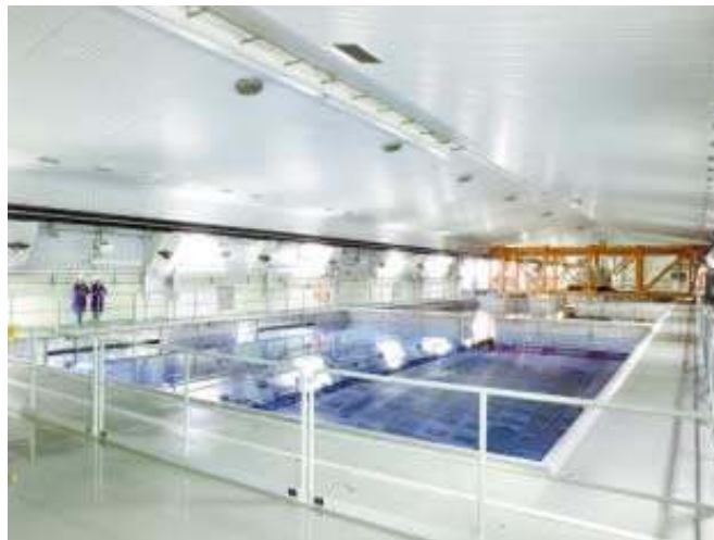
Figure 1.2.1-1 Storage water pools at the Clab underground facility, Sweden (source: www.skb.se/upload/publications/pdf/ClabEng.8.3.pdf ).
