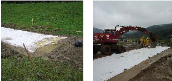
Figure 7.10: The geotextiles with applied optical cables in Solina ( left ) and Swinna Poremba ( right ).
