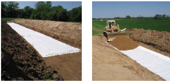
Figure 7.8: Photographs from the construction site in Dessau-Sollnitz during the first attempt to integrate sensor-equipped geosynthetics into the soil body of a river dike.
