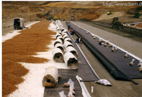
Figure 7.1: Typical application of geosynthetics: geomembranes in a composite liner system for a municipal waste landfill
