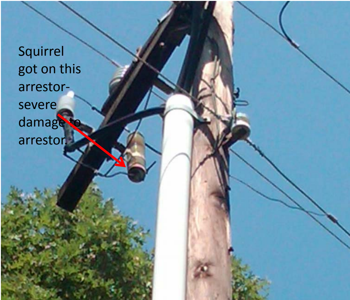
Figure 5.4: The Faulted Lightning Arrester
