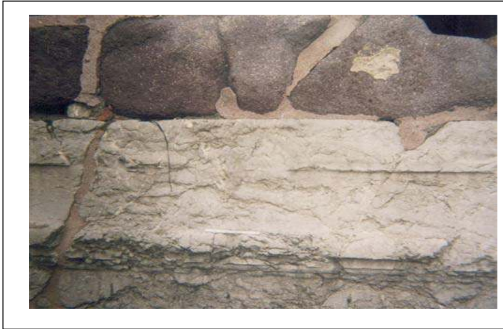
Figure 3.1 A view from west elevation at Gençkapı Gate; material loss and detachment as scales on marble surfaces
