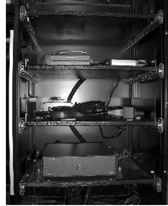
Figure 2. DieselNet equipment in a bus locker
