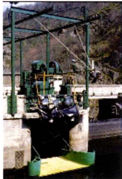
Photo 10: Surface bypass at the Poutes dam. Note the shape of the bypass entrance to create a gradually accelerating flow.
