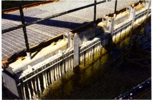
Photo 4: Surface louver screens (view from the bypass entrance) at Holyoke Canal project (Connecticut river, USA).
