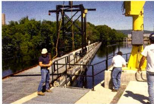
Photo 3: General view of the surface louver screens at the Holyoke Canal project on the Connecticut river (USA).
