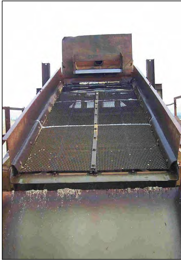
Figure 16. Screening tower with 10 mm (3/8 in.) apertures at pipeline discharge.
