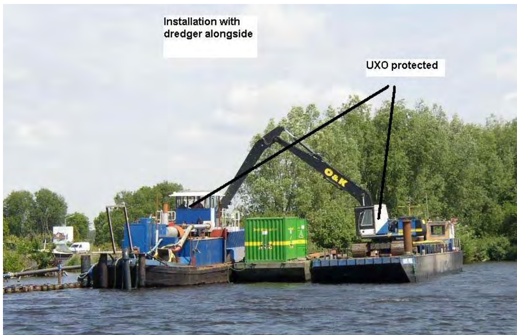
Figure 90. Armored backhoe dredge placing dredged material into separation hopper (courtesy of Heuvelman Ibis BV).
