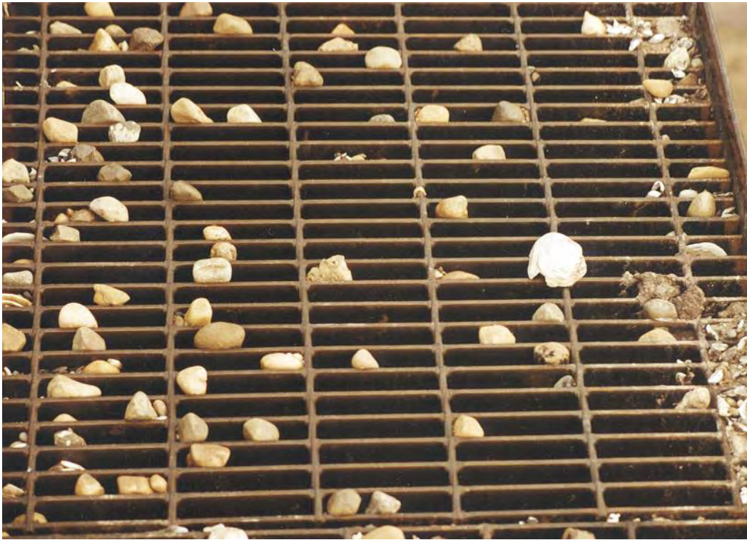
Figure 104. Blinded-off bar grate separation screens.
