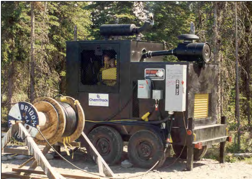
Figure 63. Diesel motor generator.
