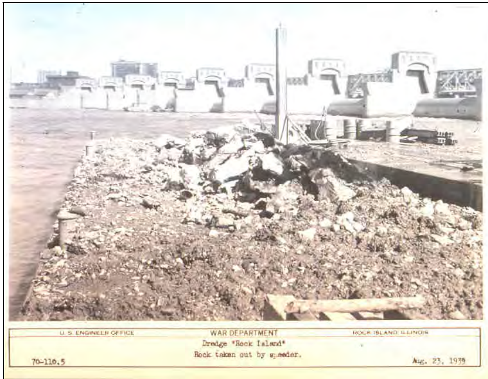
Figure 49. Sediment and rock excavated by barge-mounted dragline (courtesy of Rock Island District).
