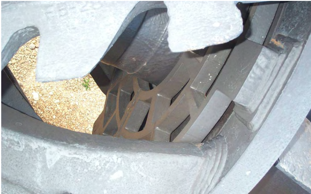
Figure 59. Closeup view of Gatling Gun suction screen (source: DSC).
