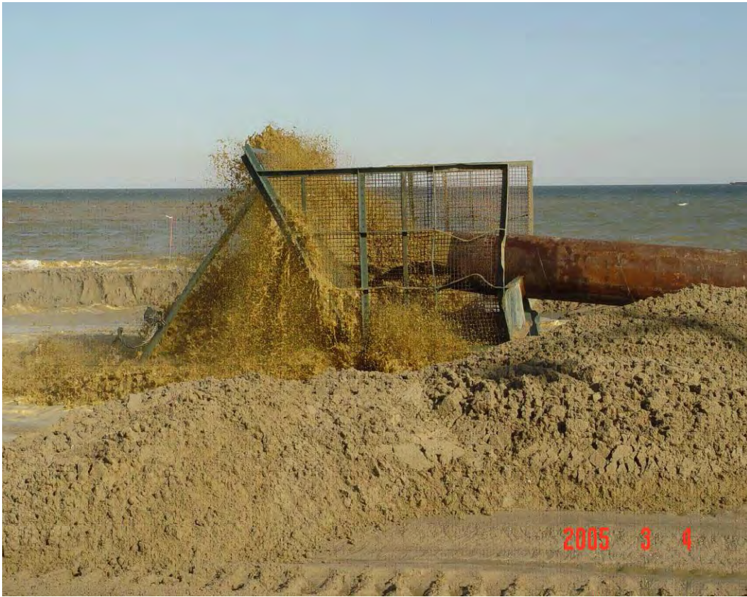
Figure 73. Discharge basket screens at Buckroe Beach.
