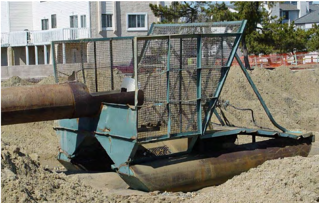
Figure 76. Discharge basket screen ready for next filling cycle.
