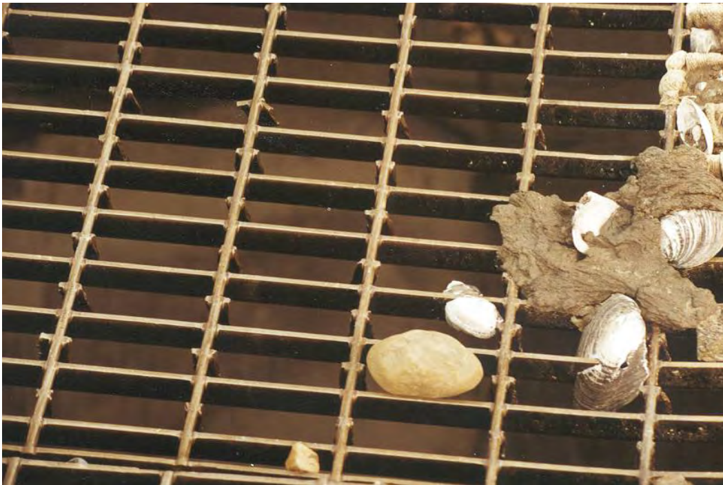
Figure 105. Modified bar grate screens.
