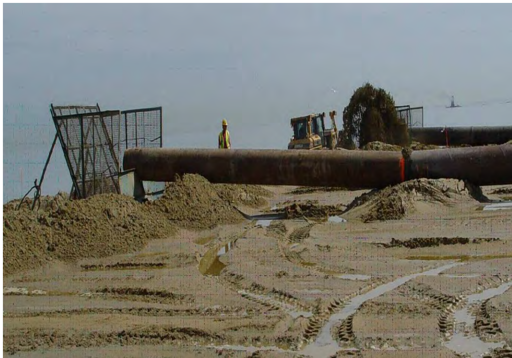
Figure 74. Two discharge basket screens on a bifurcated discharge line.
