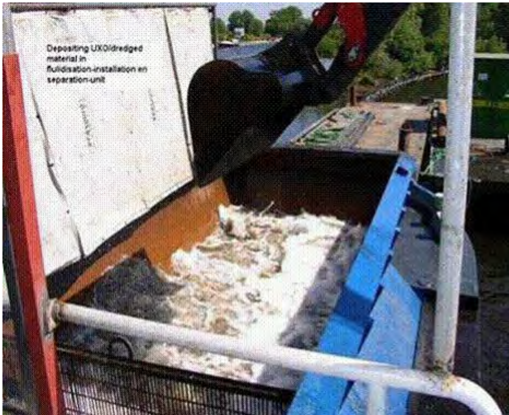
Figure 91. Closeup of bucket placing MEC-contaminated material into separation hopper (courtesy of Heuvelman Ibis BV).
