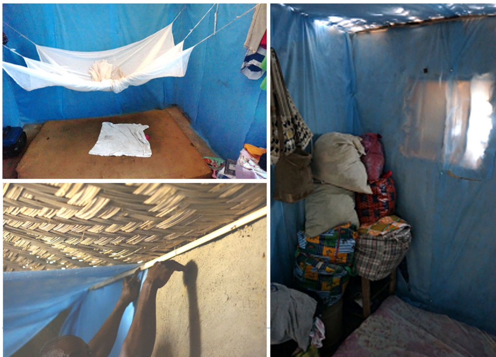
Fig. 4 Photos of typical installation of DWL in houses in Bomi County, Liberia. Deltamethrin LLINs were present as an additional control measure in both arms of the study. Ceilings and windows were covered with DWL using wooden strips
