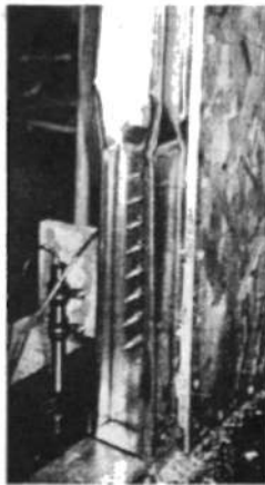
Figure 8 Crippling in chord stud
