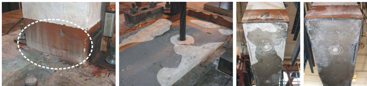
Figure 13: Damage state after removal of the precast wall from the foundation; Left: Dust flume on steel confining plate indicating expulsion of crushed concrete, Left Centre: Foundation recess with residual concrete, Right Centre: Rocking toe region (closest to mass), Right: Rocking toe region (furthest from mass)
