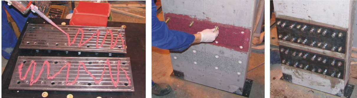
Figure 9: Damper connection details; Left: Preparation of the steel plate – roughening and application of high strength epoxy, Centre: Roughening of the concrete, application of high strength epoxy and location of the high strength threaded rods, Right: Installation of the steel plates - threaded rods tightened to 65% proof load.
