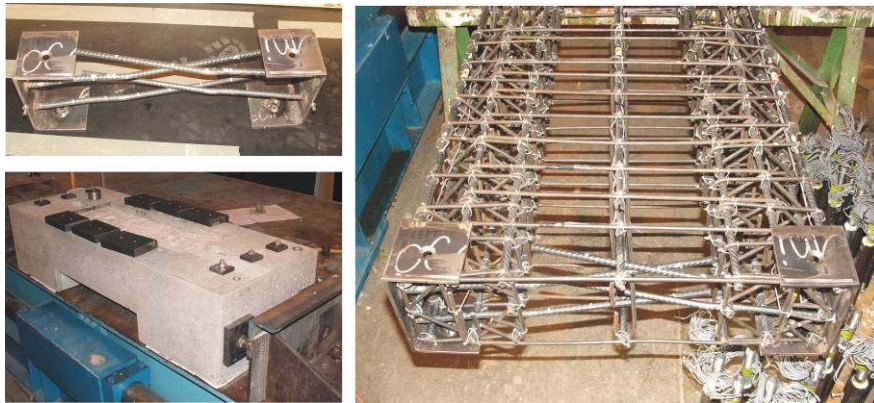
Figure 7: Construction of the precast wall unit and precast foundation; Top Left: Steel confining plates, Bottom Left: Precast foundation, Right: Wall reinforcement
