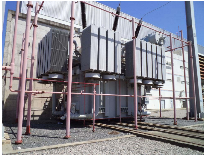
Figure 11. 29 MVA transformer of Termopernambuco Thermal Power Plant.
