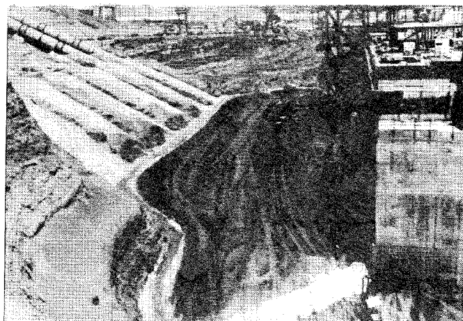
FIGURE 2: CASTAIC POWER STATION UNDER CONSTRUCTION, SHOWING SOIL BACKFILLING BEING PLACED AGAINST WALL OF STRUCTURE.
