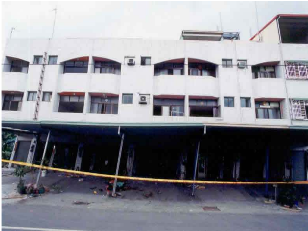
Fig. 1.3: General mode of failure in OGS buildings
