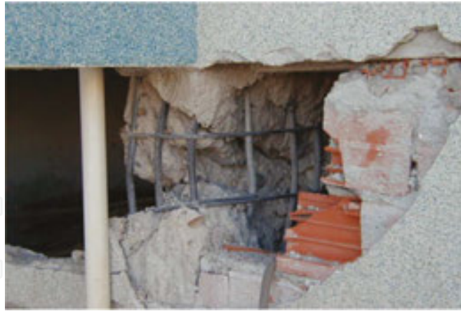
Figure 13. Short column damages during the 2003 Bingöl earthquake.
