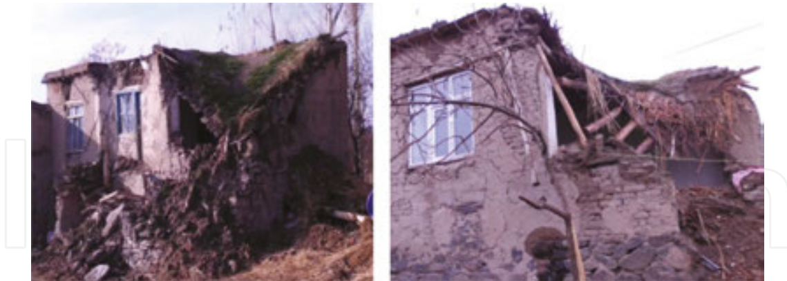
Figure 19. Damage to adobe structures due to heavy earthen roof during the Van earthquake [42].
