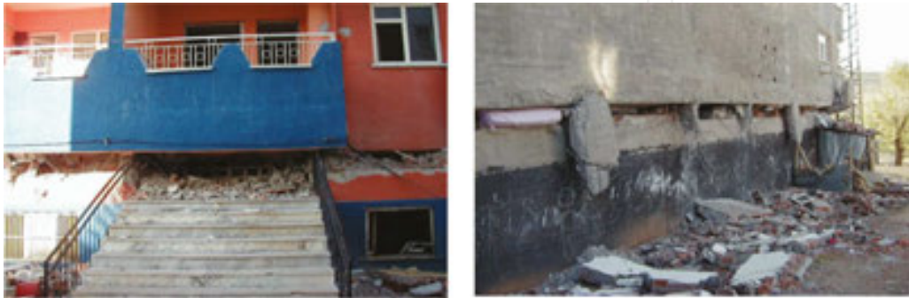
Figure 11. Weak storey mechanism during the Bingöl earthquake.
