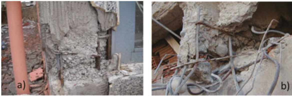
Figure 17. Failure of column due to poor concrete quality during; (a) Van earthquake and (b) Bingöl earthquake.
