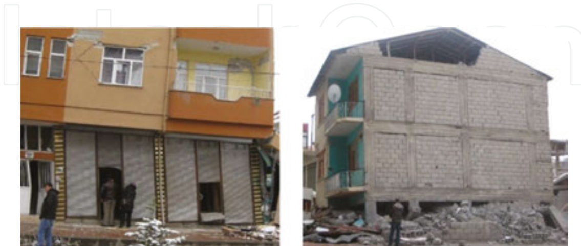
Figure 10. Unexpected inter-storey drift due to soft storey during the Van earthquake.
