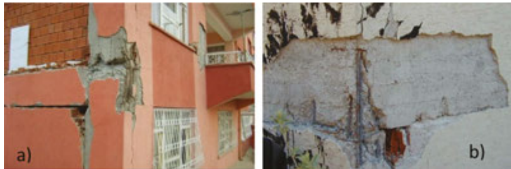
Figure 12. Damaged structure due to inadequate spacing between shear reinforcements during (a) Van earthquake and (b) Bingöl earthquake.
