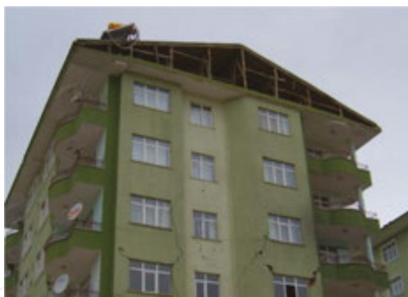
Figure 16. Failure of gabble walls on top of the building during the Van earthquake.
