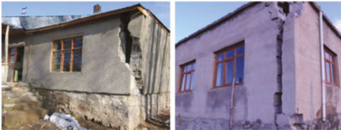
Figure 20. Corner damage of briquette masonry buildings [42].
