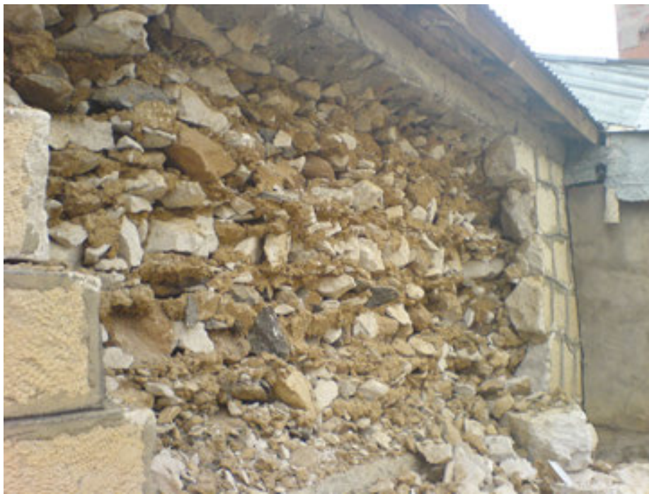
Figure 23. Disintegration in stone masonry buildings [28].
