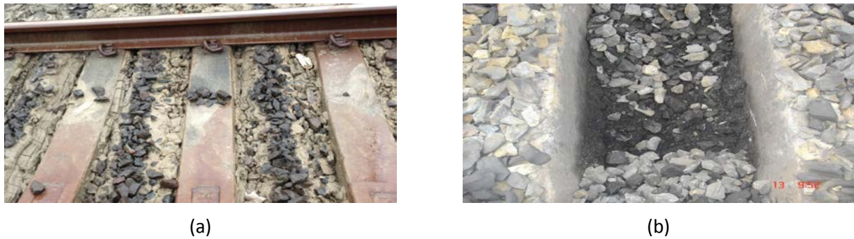
Figure 2: Ballast contamination due to (a) clay pumping in Ashfield, New South Wales, Australia and, (b) coal contamination in Rockhampton, Queensland, Australia
