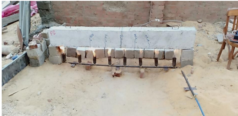
Fig. 25: During the fire for the beam (F-G).
