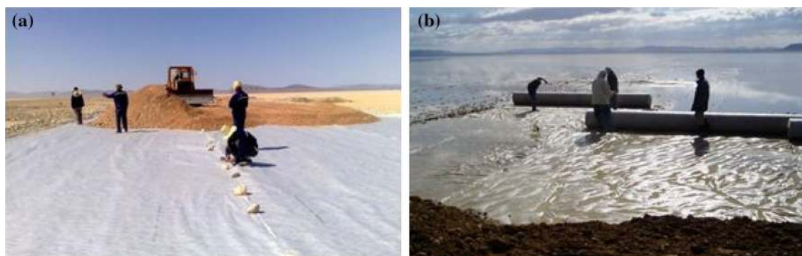
Fig. 6 Laying directly over sabkha surface a nonwoven geotextile. a Dry state. b Flooded state
