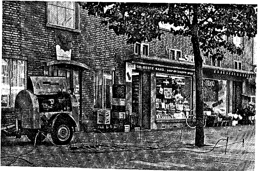
Fig. 32. Compressor treatment near a tree affected by gas leakage (photograph VEG-Gasinstituut, Rijswijk).
