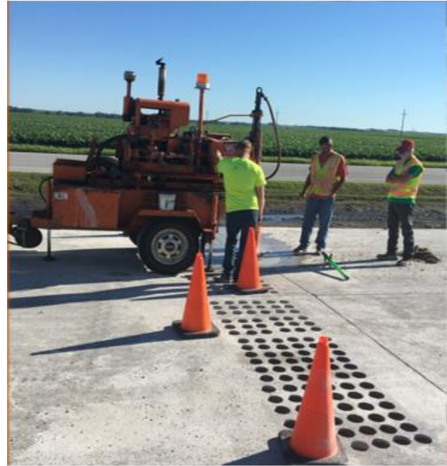
Figure 1 - The coring crew cuts research cores in a grid on the Hwy 30, Schuyler-Rogers project.
