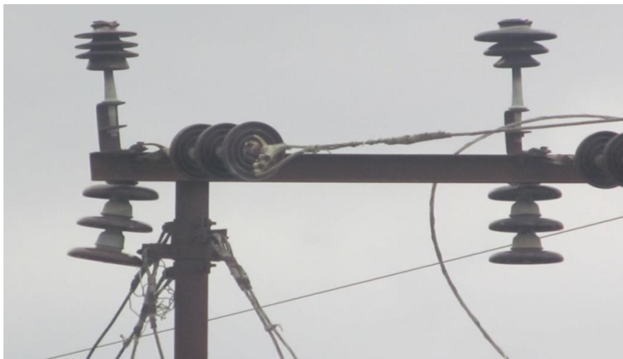
Fig. 10: Coated and Uncoated Post Insulator Was Kept at Dead End Electric Pole of 33kv Hot Line.
