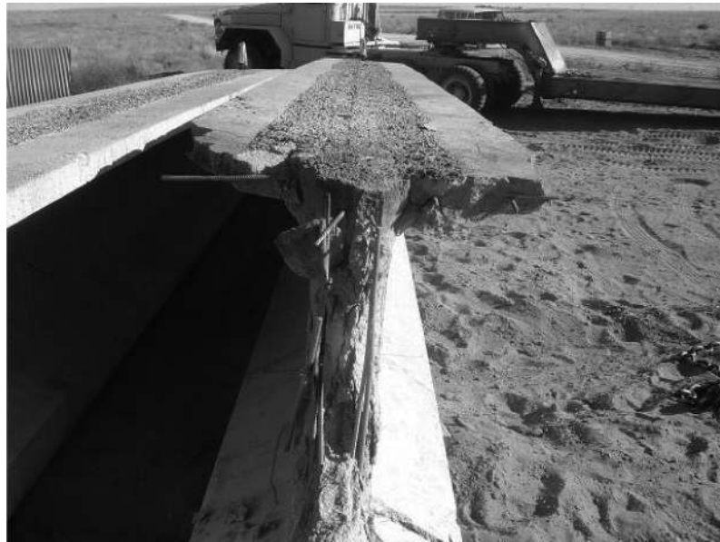
Fig. 9. Web cracking from blast above the girder.
