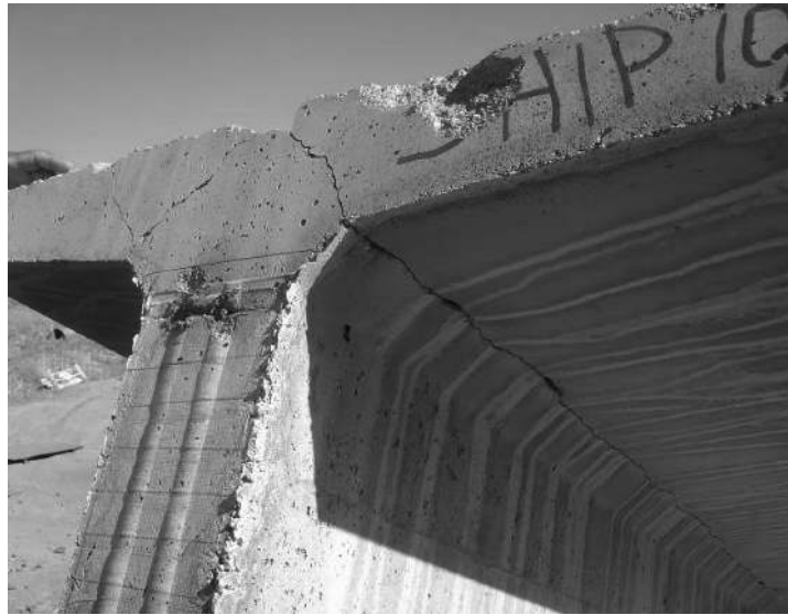
Fig. 13. Longitudinal cracking at web-flange intersection.
