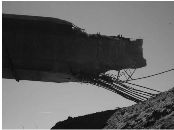
Fig. 15. Damaged section with rubbelized concrete removed (adopted from [12]).
