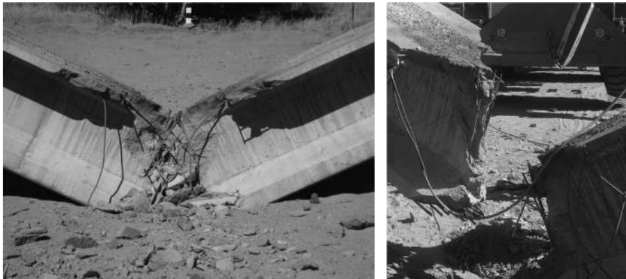
Fig. 7. Damaged girder from blast above midspan (adopted from [13]).
