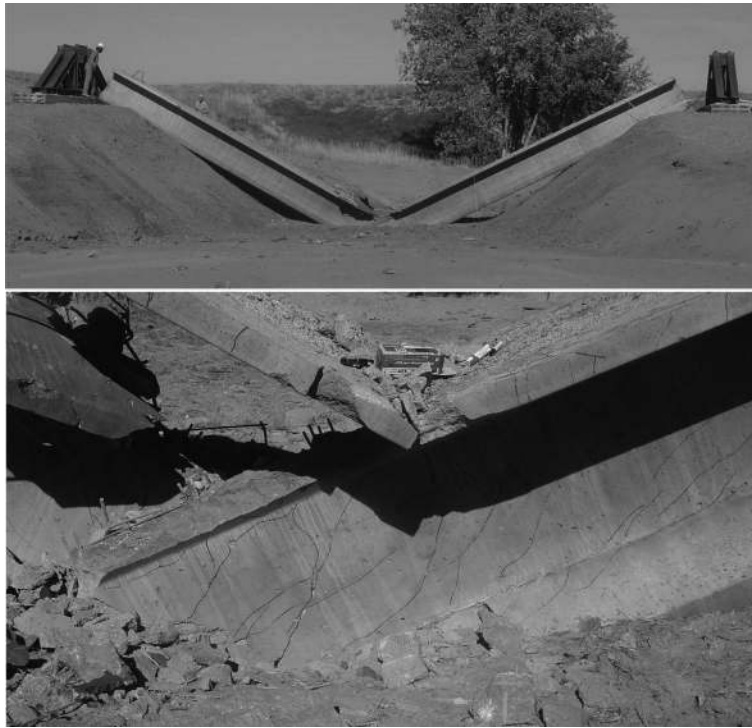
Fig. 12. Damage from the blast below the girder.
