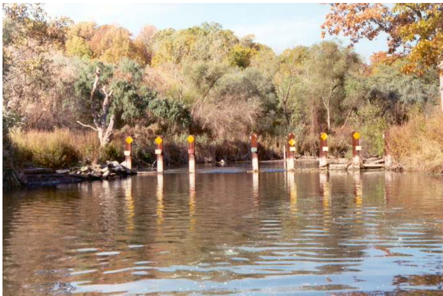
Figure 5. Schematic diagram and photograph of flow-control structure at the Narrows in Ellison Park wetland, Monroe County, N.Y., 2001. A. Schematic diagram. B. Downstream-facing view of flow-control structure with H-piles extending above water surface.
