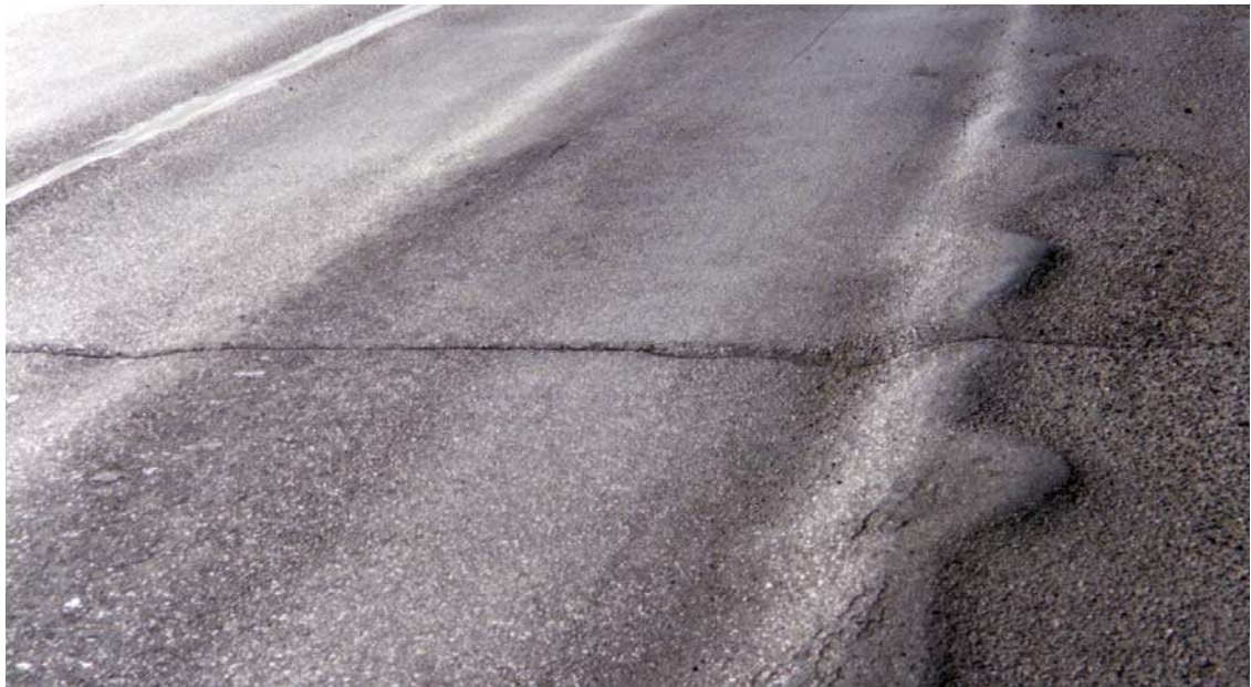
Figure 2.4 Visco-plastic Rutting in Asphalt Pavement Layer (courtesy Dr. C .F. Berthelot)
