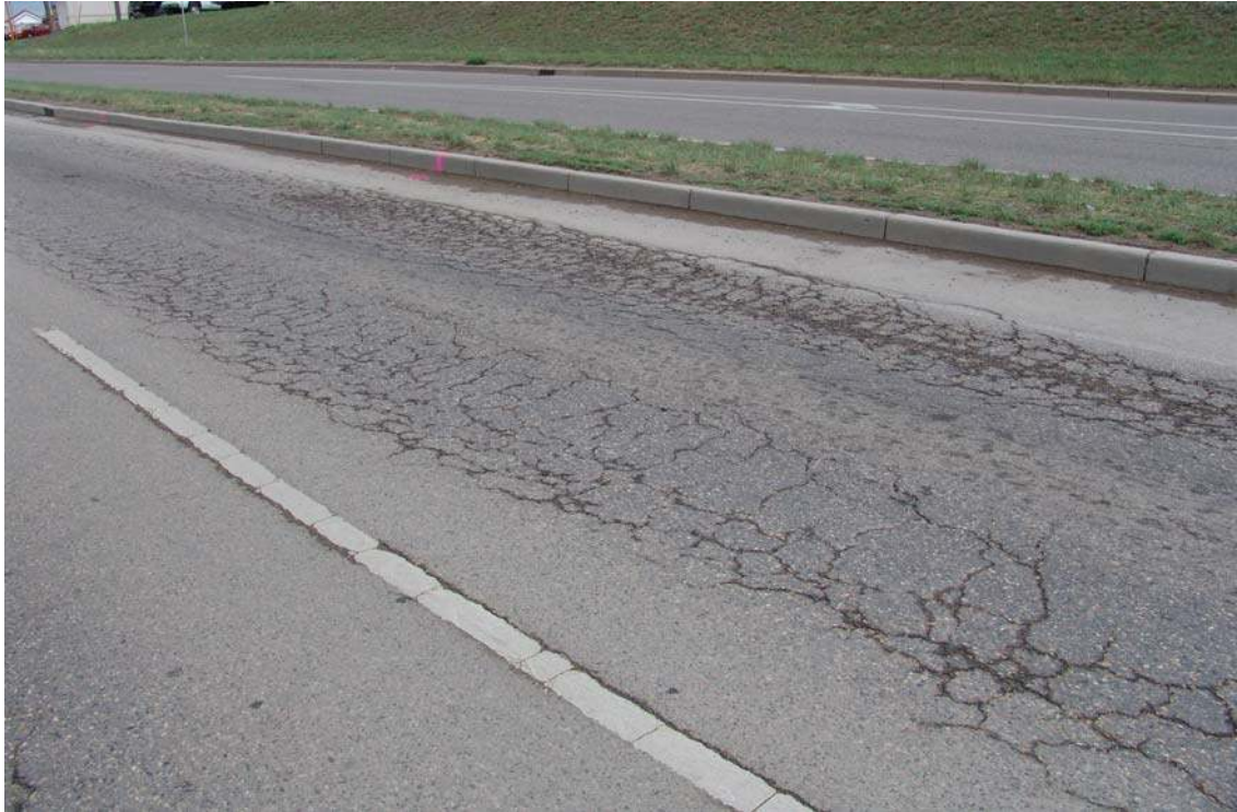
Figure 2.2 Structural Rutting (courtesy Dr. C. F. Berthelot)
