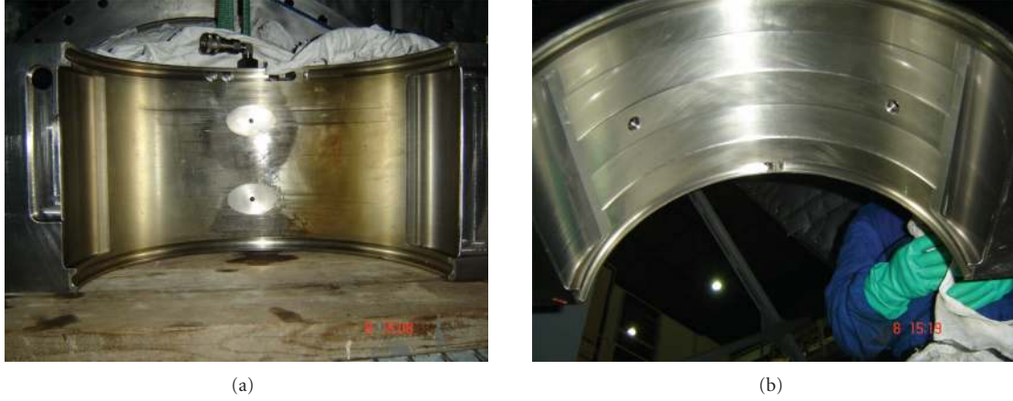
FIGURE 6: Visual inspection of bearing no. 1: (a) lower lobe and (b) upper lobe.
