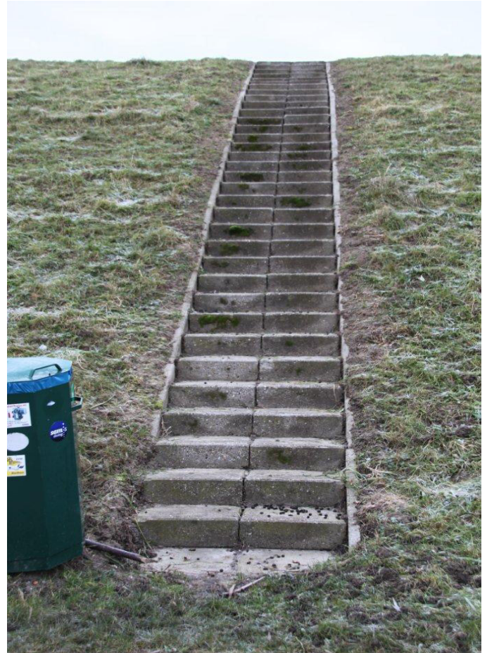
Figure 2.2 Patchy turf; Tholen, Section 2, Stair (before testing)
