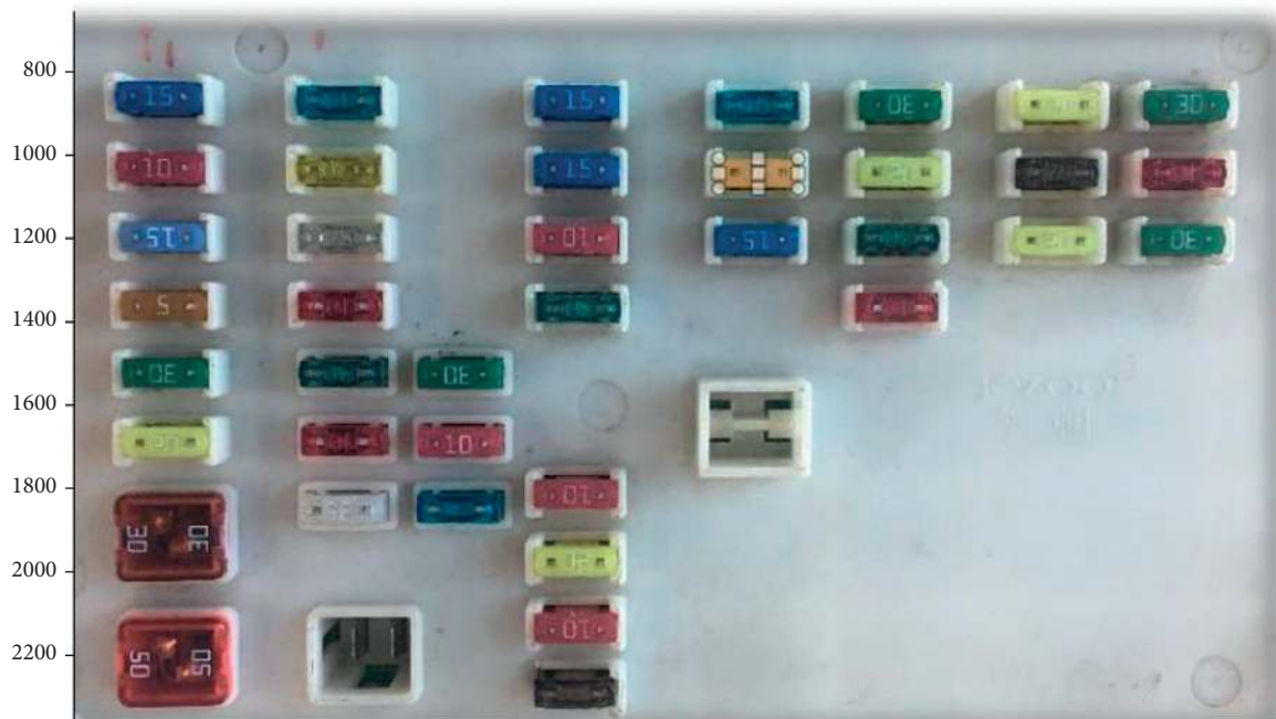
FIGURE 6: The fuse board.
