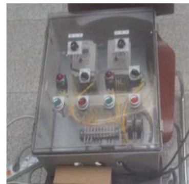
(b) Control box
