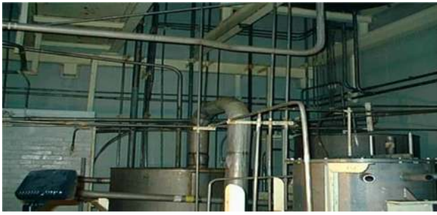
Fig. 1 Photo of pipework from an exemplar facility
