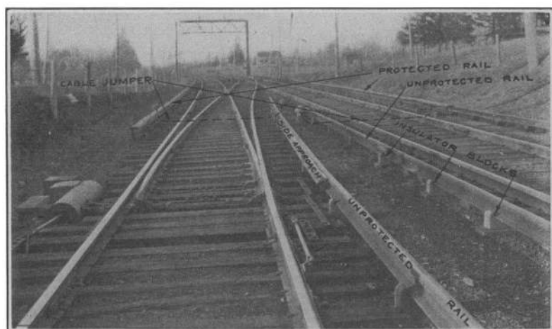
FIG. 8.—Third rail at cross-over
