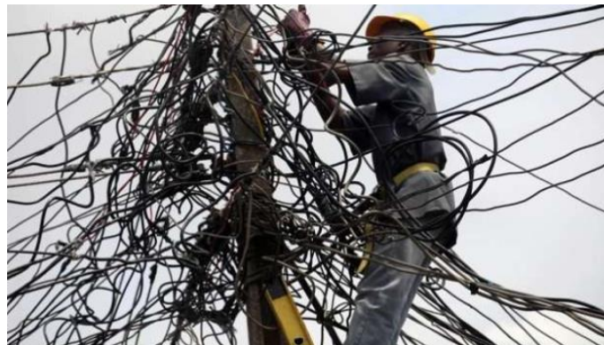
Fig. 1: Electricity Theft by Direct Connection to the Distribution Feeder [21].
