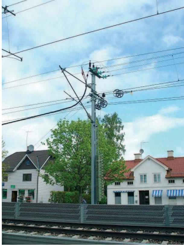
Figure 6.1: Cable termination at the auxiliary power conductors
