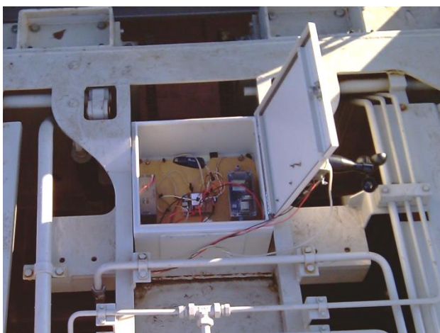
Fig. 1. Data logger attached to one of the train carriages for vibration measurement.
