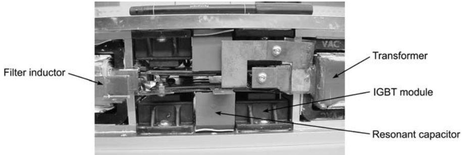
Figure 5-4: Integration of converter components, view on bridge modules with filter inductor on the left and transformer on the right side
