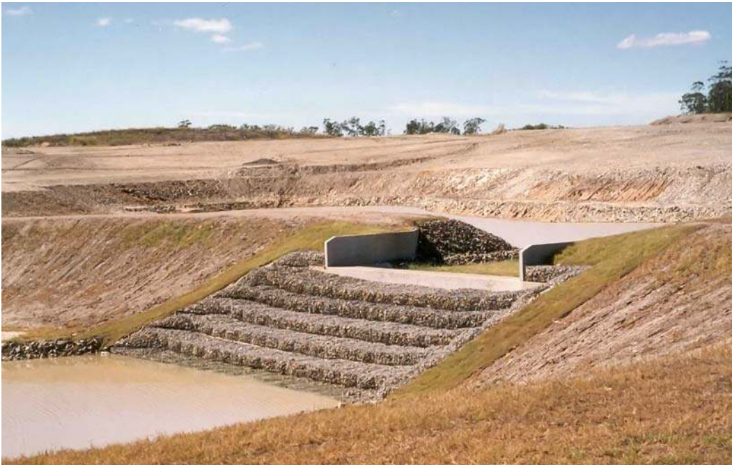
Fig. 7 - Gabion weir: Robina stepped weir No. 1 (Gold Coast, Australia) on 2 April 1997, shortly after completion: h \sim 0.5 m, h/l \sim 0.5
