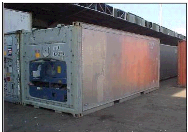
Figure 1. Reefer refrigeration system
