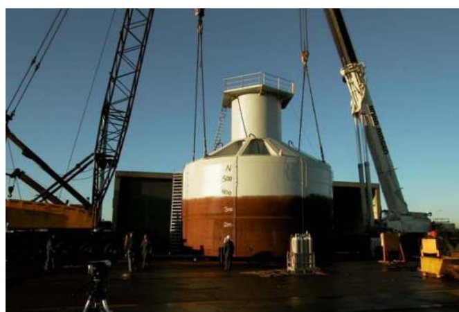
Fig. 3. Bucket foundation for the Vestas 3-MW wind turbine in Frederikshavn (reprinted from Barari 2012, with permission)
