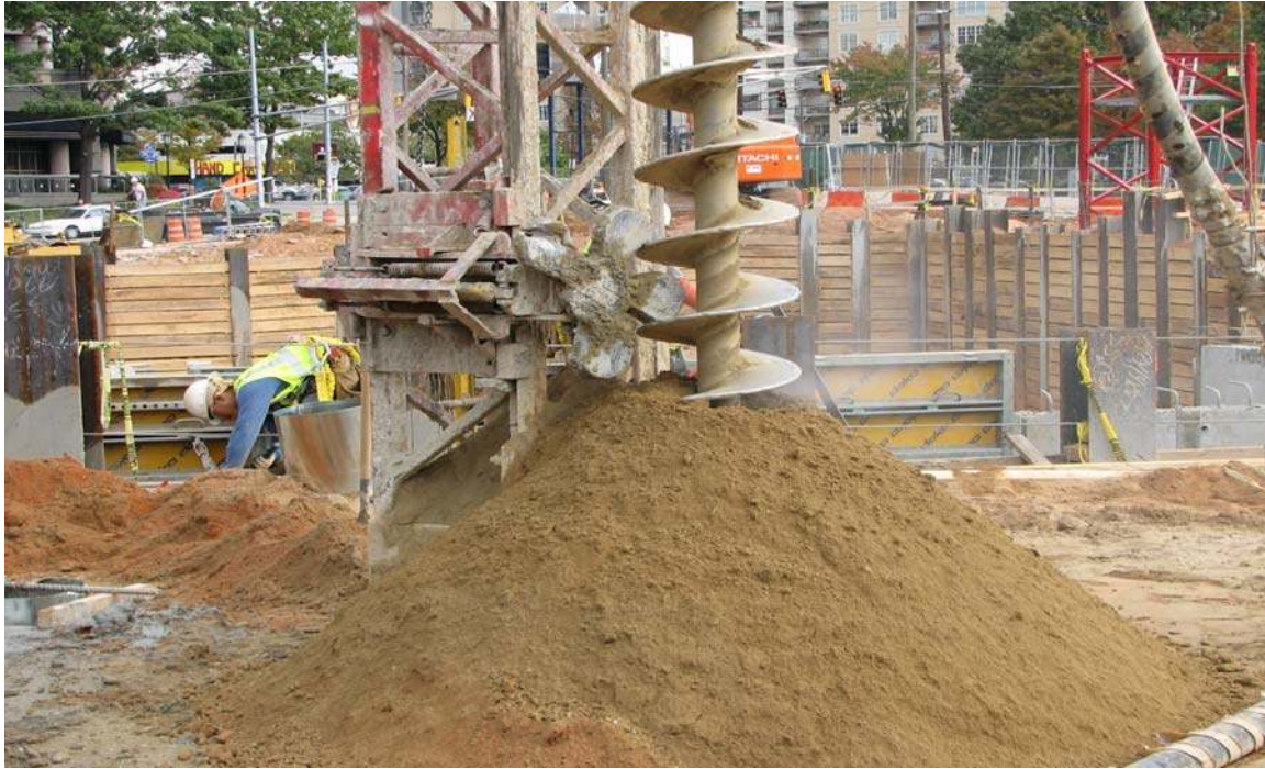
Figure 37-Picture of auger removing soil to begin pumping of grout to cast pile.
