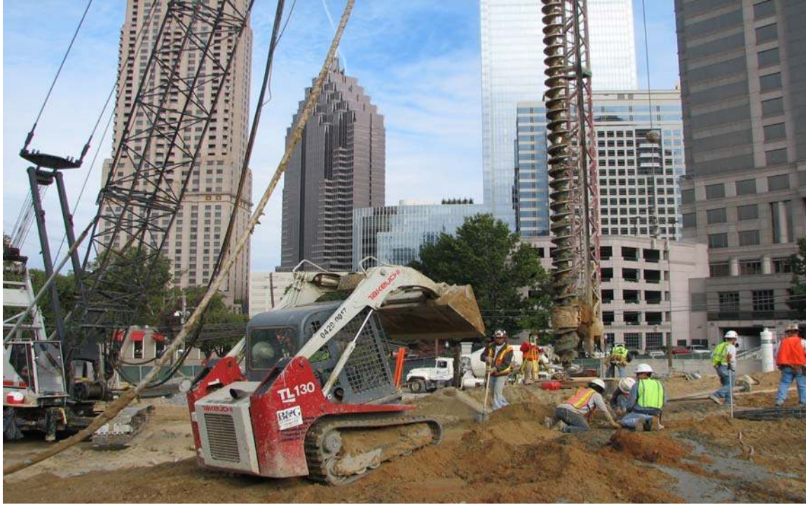
Figure 35- Picture of hollow stem auger, crane, and leads after placement of grout pile.
