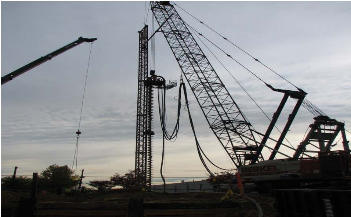
Figure 36- Picture of installation of grout pile with hollow stem auger and crane.
