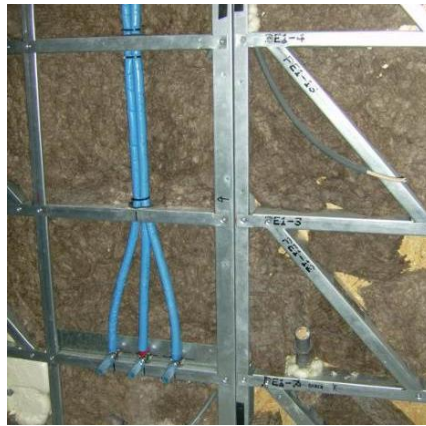
Fig. 2. Technical installations between steel frames.
