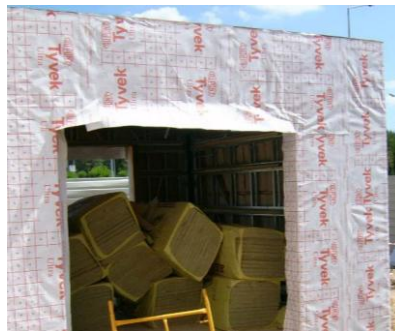
Fig. 5. External wind-tightness membrane layer around an opening in a LSF external facade before the ETICS execution.
